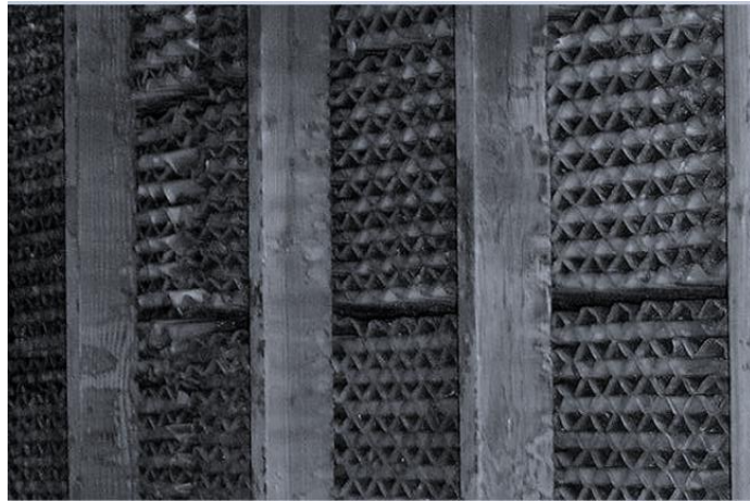
Clean cooling tower
